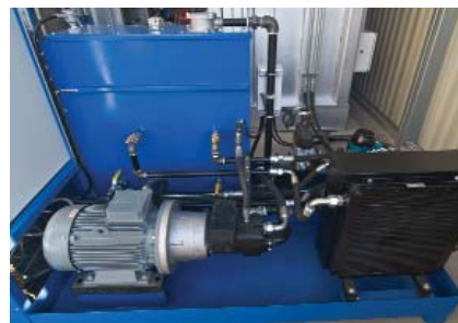
2 Hydraulic system of the new TARDIS Generation 2 press.
