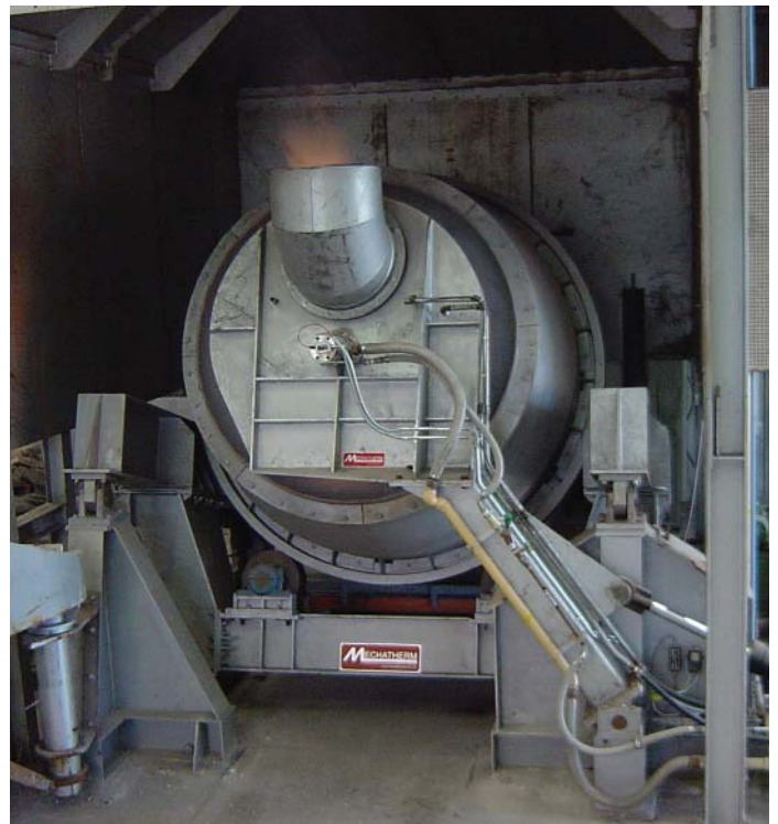
Mechatherm International 5 tonne tilting melting furnace
