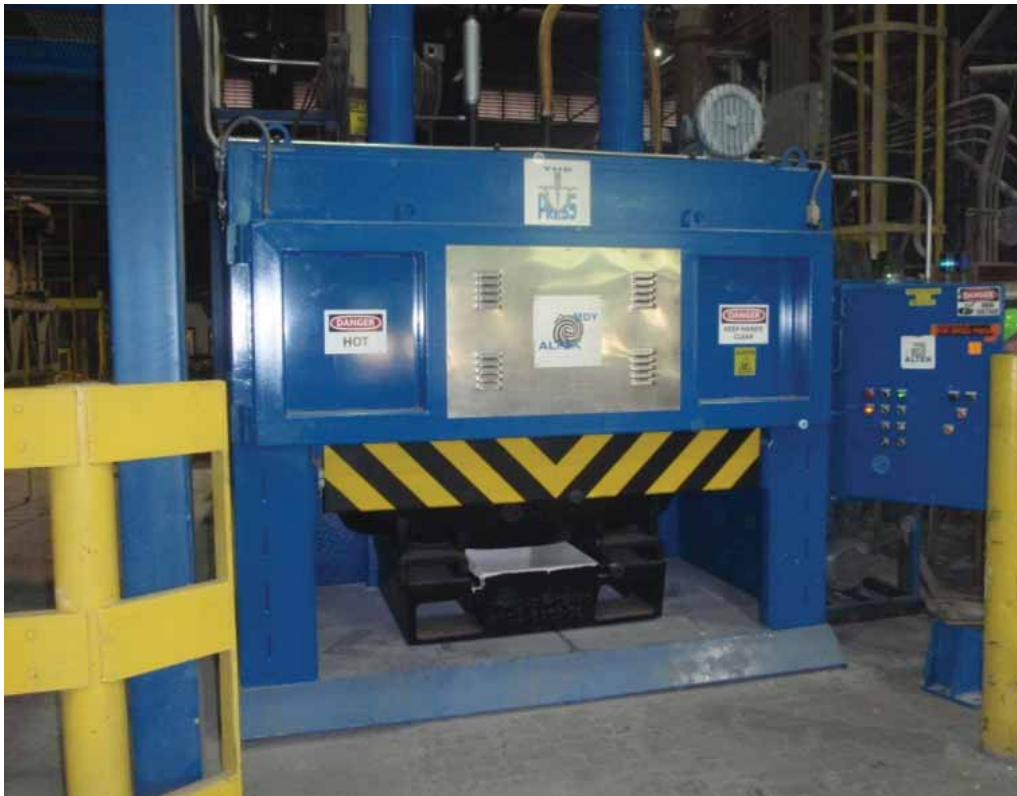
Rebuilt dross press showing the automatic safety shield door
